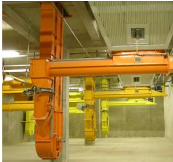
Foot above ground with optimized discharge
