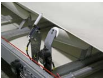
Belt misalignment control
