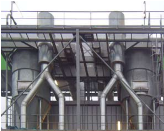
Sleeves filters with decoupling valves, explosion vent
