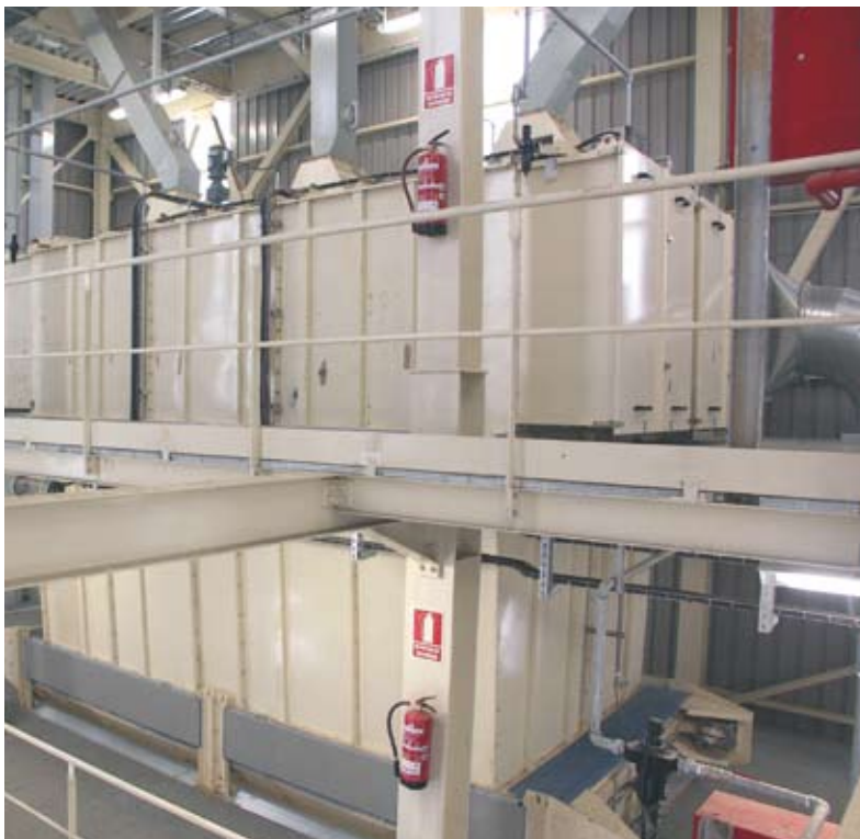
Pads filter on cooler
