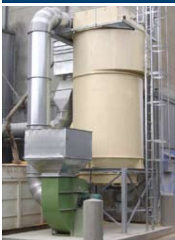
Sleeves filters with rotary extractor
