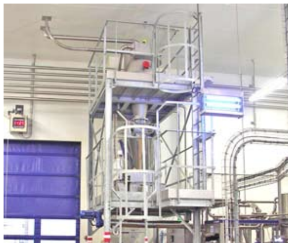
A pneumatic conveying feeding by a cyclone
